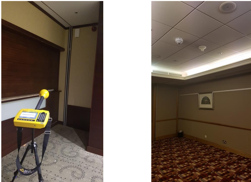
Figure 2 – Peak Measurement Location with wall-mounted antenna in background (left) and ceiling-mounted antenna in adjacent room (right)
